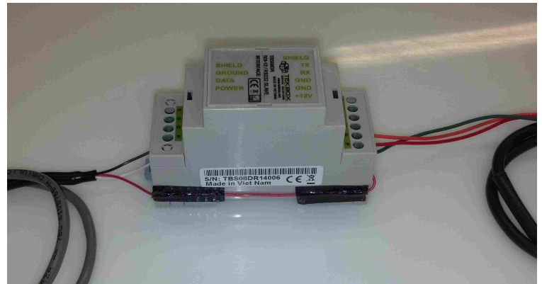
Fig. 7: ProbeGuard SDI-12 convertor showing +12V supply wire along side of unit
